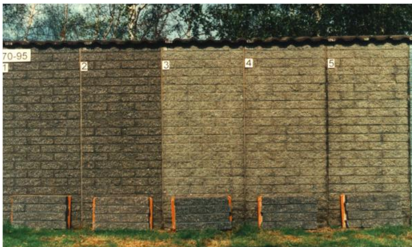
Photo 7: Concrete masonry blocks (unweathered reference samples in foreground) Weathering commenced: 1970, Photo taken: 1995
