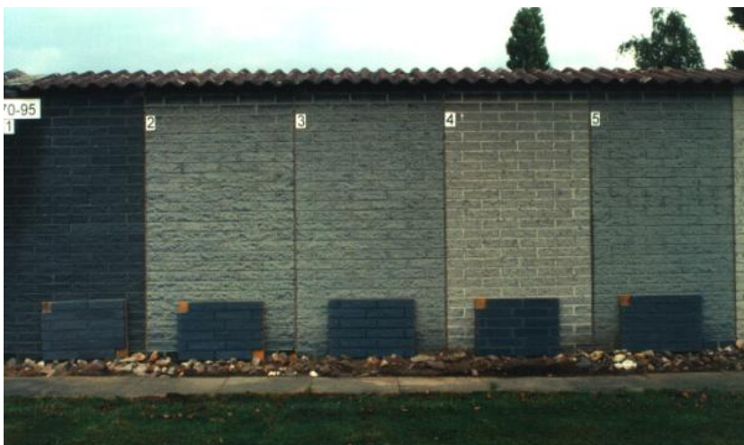
Photo 8: Calcium silicate bricks (unweathered reference samples in foreground) Weathering commenced: 1970, Photo taken: 1995
