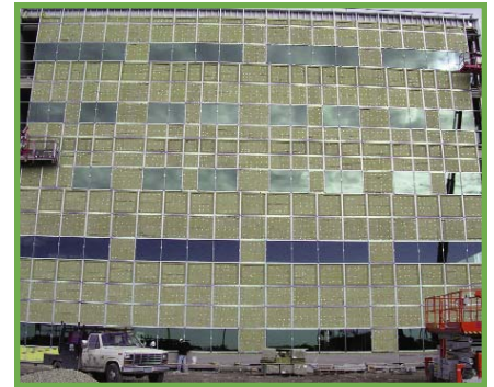
This facade shows insulation pin welded to back pans prior to being covered with metal wall panels. Alberta Children's Hospital, Calgary, Alberta. Kasian Architecture.
