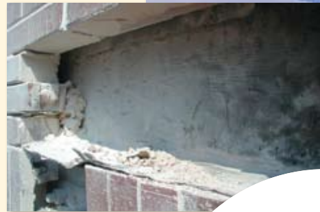
Pictured above is a wall failure due to excessive mortar build up in a cavity wall.
