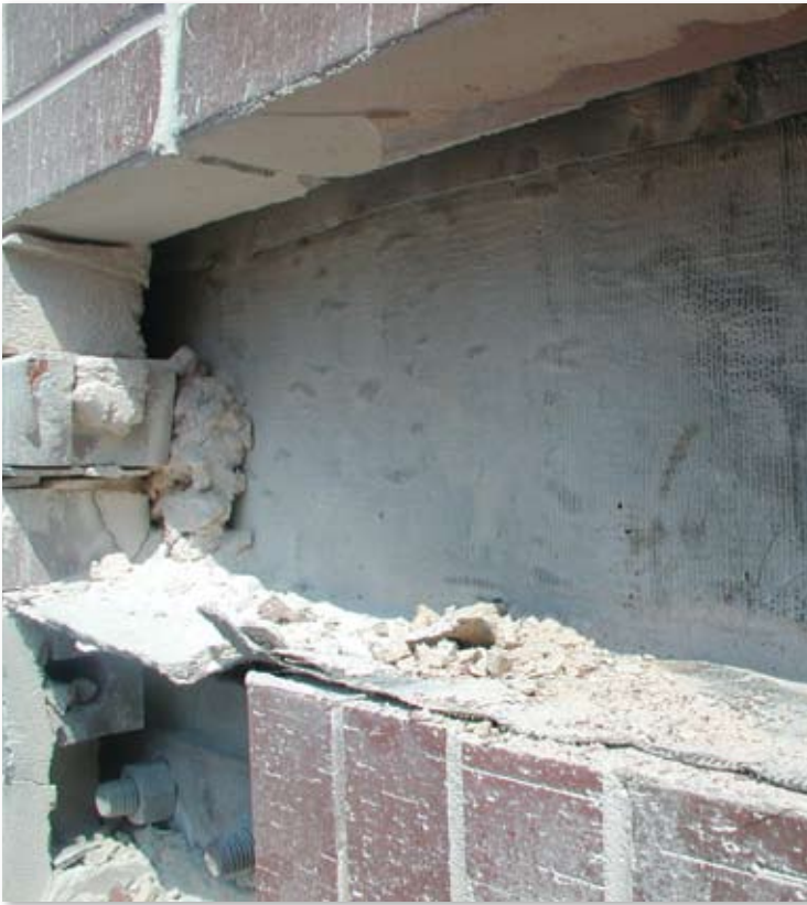
Above picture is a wall failure due to excessive mortar build up in a cavity wall.
