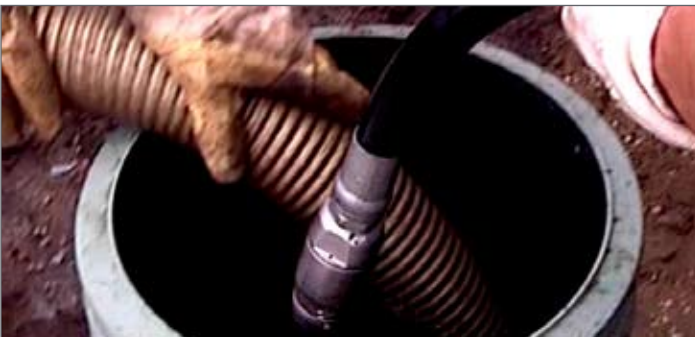
Figure 9: A pressure hose and flexible vactor hose are lowered into the Stormbloc™ Inspect access port
