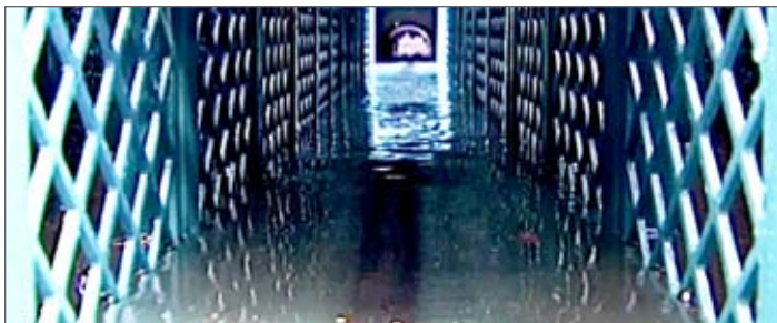
Figure 11: The vactor hose draws the water and loosened debris out of the Stormbloc™ system
