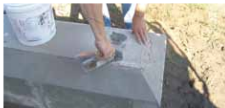
Prior to sign placement, utilize the provided sign setting kit, including mortar, trowel and mixing pail to fill preformed pockets in the footings.
