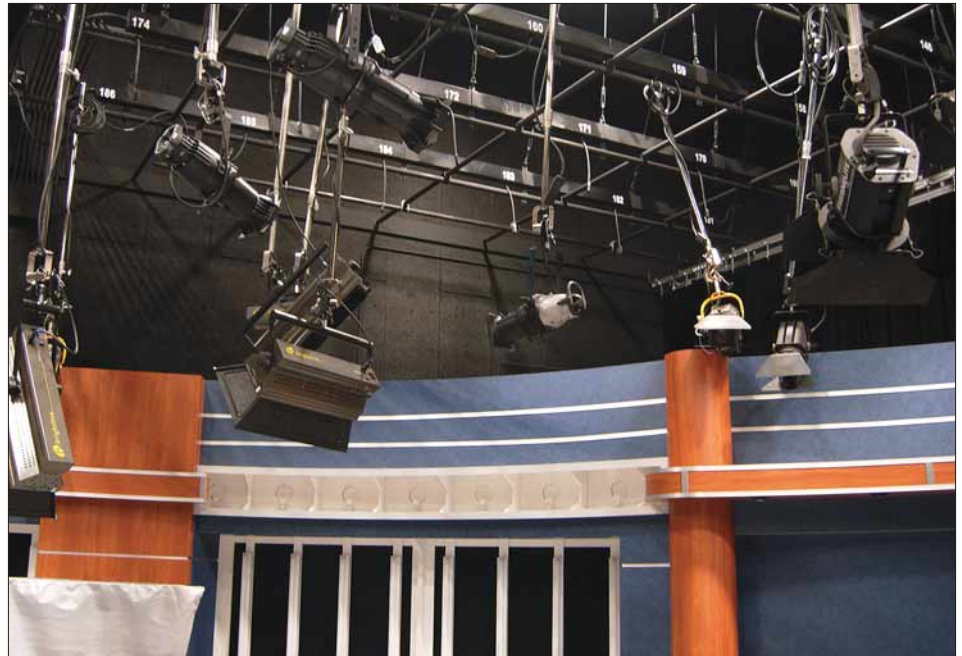
Broadcast systems can be designed to read as low as NC15 with a reverb time of .75 seconds .....guaranteed.
