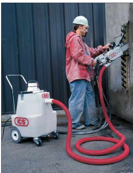
70% slurry containment using (TSS™) products as a system with an ICS 853 Pro Series saw
