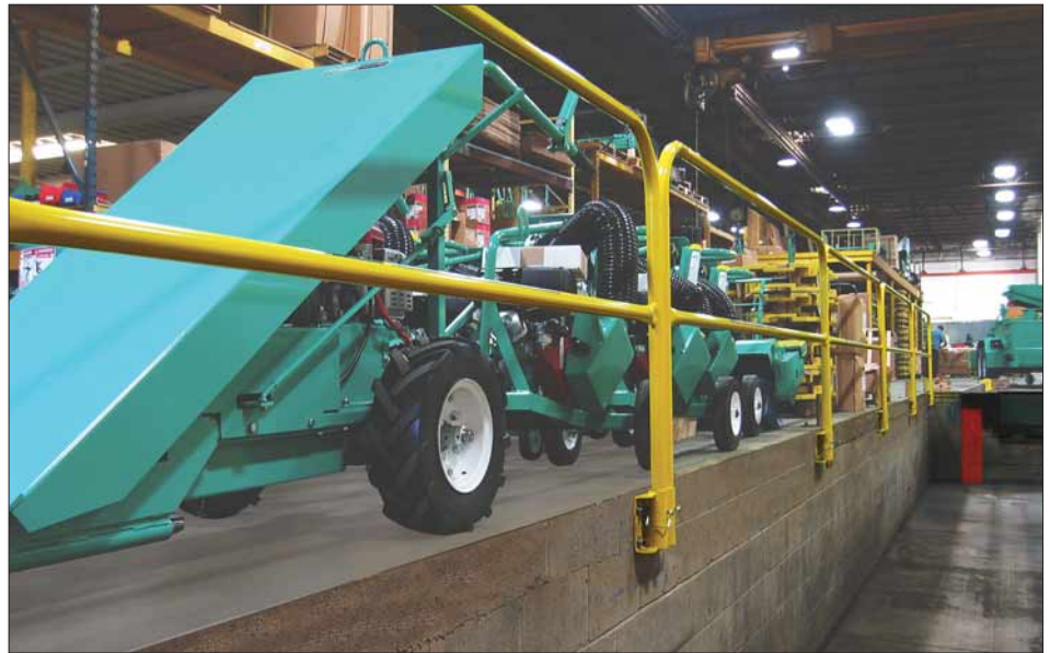
Shipping pit with permanent sidewall mounting brackets and quick-release pins that allow rail sections to be removed when access is required
