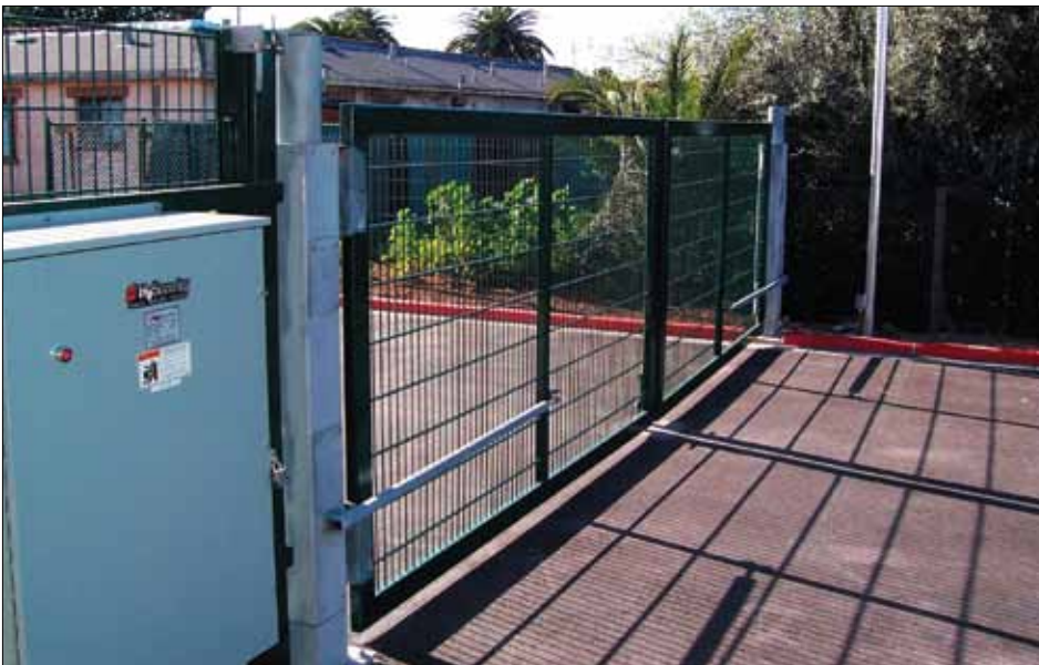
Separate electrical enclosure (left) operates both gate panels in unison in this SwingRiser Twin configuration.
