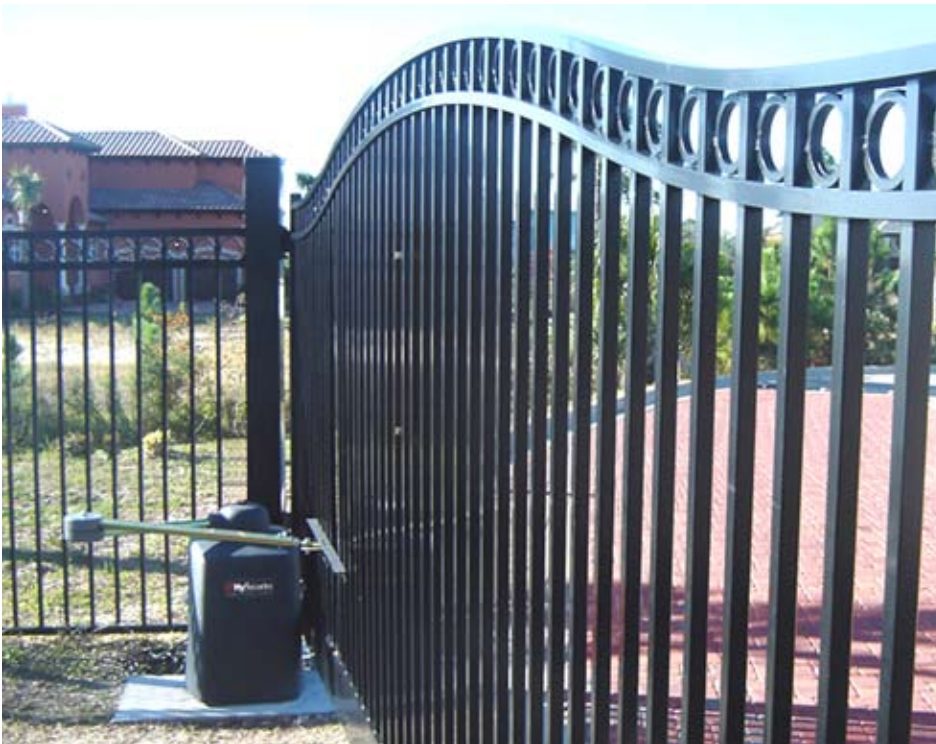
SwingSmart DC 20 reliably operating at a condominium complex along the salty and humid Florida coast.
