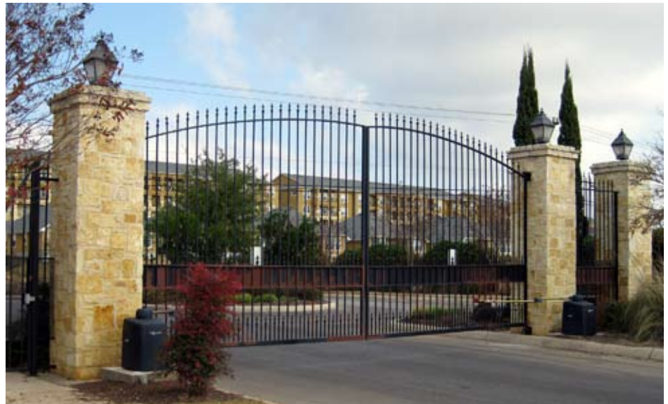
Dual SwingSmart DC 20 gate operators installed on Arizona private estate. Each 16' (4.87 m) ornamental iron gate weighs 800 lb (363 kg).
